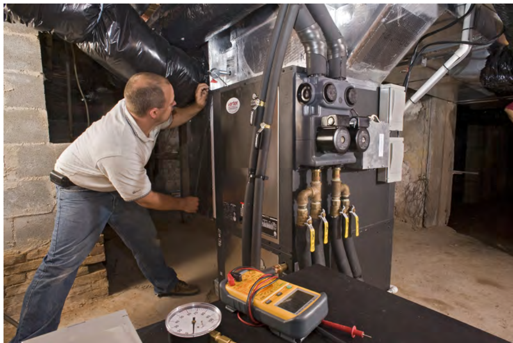
Vince Youndt performing a routine service check on the system (above) as well as its air handler section (below).
